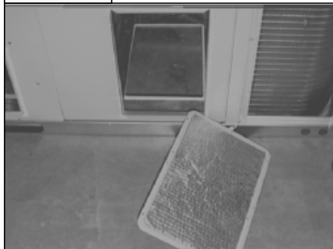
Blockoff Plate Removed (Return Air Compartment)
